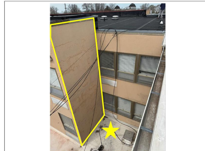
Similar to what we see below the arched stone caps, the wall on the left has obvious water damage and evidence that it could be debonded. It should probably be replaced. This is also an area where the office leak was reported. We should inspect the wall and the roof transition details to better understand what is going on here.
