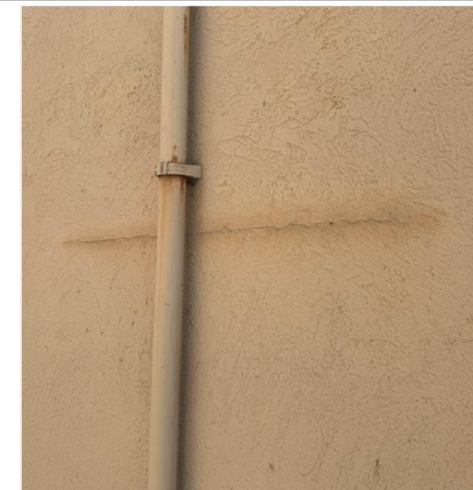
This fracture along an EPS insulation board joint has allowed water to penetrate which is exhibited by the dark coloration around the crack.
