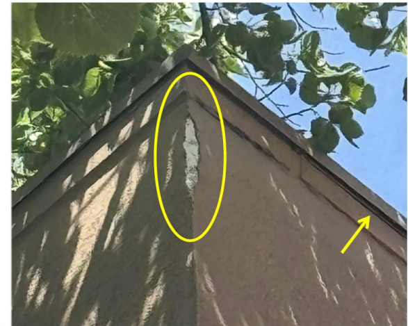
This is a typical tree scrape where a chunk of the system has been ripped away leaving exposed insulation. This should be fixed before winter. It also appears that there is a failing sealant joint at the top of this wall. We need to get a closer look.
