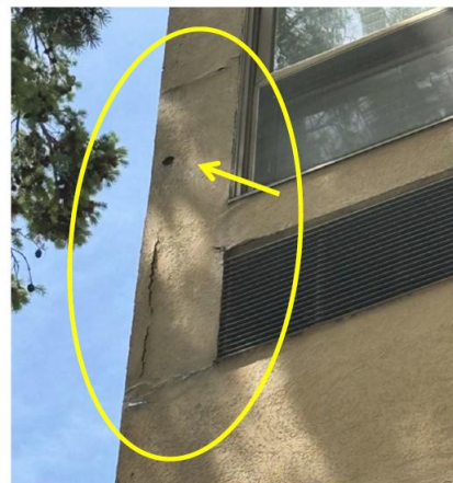
Fracture with large gap, poorly repaired. Also a bird hole above it. This entire area is an issue and should be repaired before winter.
