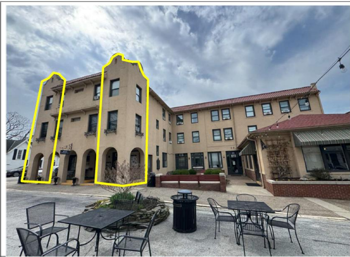
Overview of east façade. Concentrated concern areas are highlighted. Typically, these are below the arched caps.
