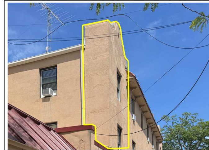
Notice the system to the left of the downspout is in much better condition. More evidence that the stone caps are the culprit.
